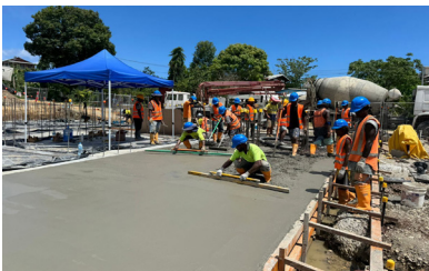
Concrete slab and foundation works at the Naha Birthing and Urban Health Centre.
