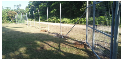
Work progressing on the installation of a fence around a health clinic in Rennell and Bellona, funded through the Solomon Islands – Australia Community Partnerships.
