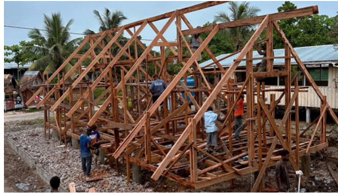
Construction of a FaeFae (kastom haos) in Lilisiana, Aoke/Langalanga designed to be a community meeting hall for chiefs to pass down traditional knowledge, funded by Australia.
